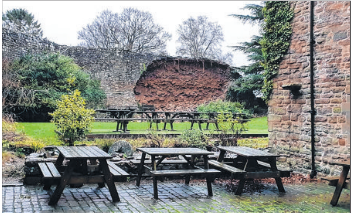
A large part of the moat wall at St Briavels Castle fell last week, following heavy rain
